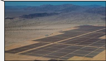
Dedicated Solar plant outside the Port Zone (80 MW)
